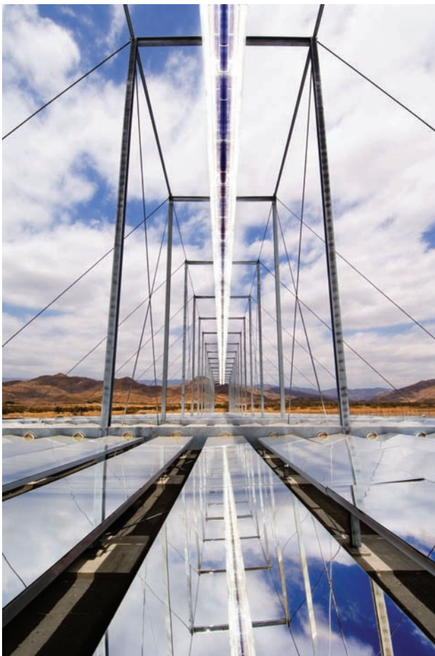
Figure 3.3 Solar receiver for Linear Fresnel technology (DLR, Markus Steur).
